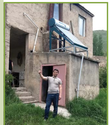
Installation of solar water heater on the roof of Meghradzor Educational and Cultural Center
